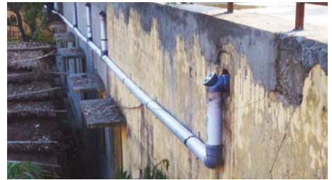
Rain water pipe connection from roof to filter
