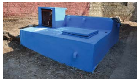
Under ground water storage tank
