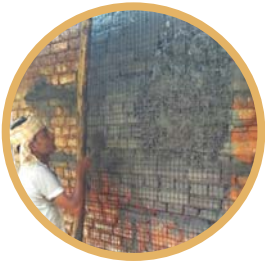
Strengthening of wall junctions and corners with steel reinforcements, wire mesh jacketing and polymerized cement plaster
